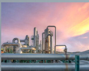
OIL & GAS FACILITIES
